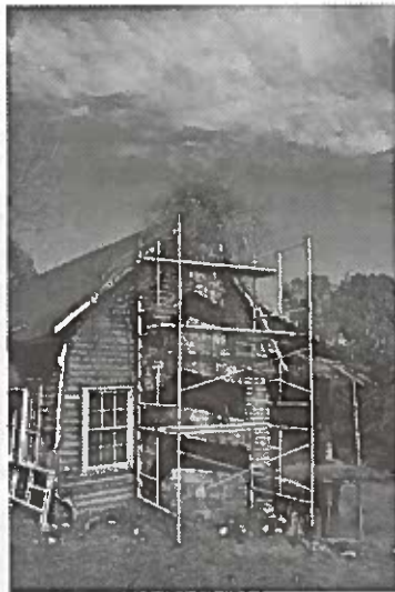
Stone mason David Vandiver stabilized the chimney that was falling into the cabin. He will reassemble the chimney to its original form.
