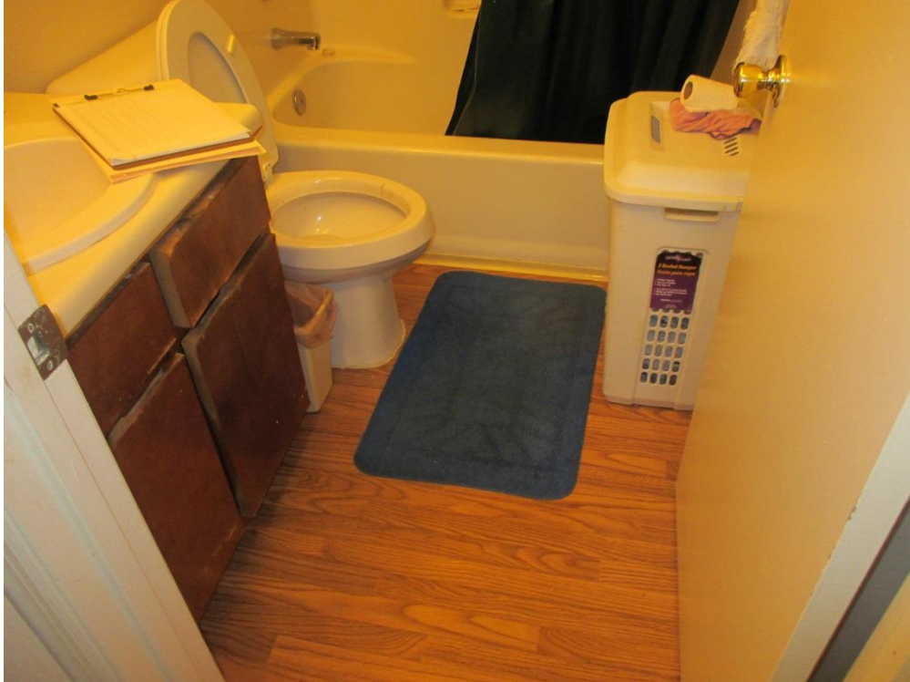
View of Bath - One-Bedroom Unit
