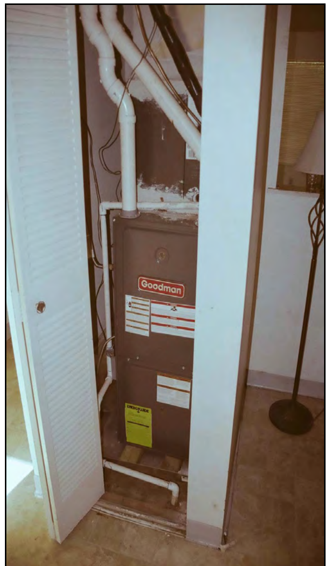
(12) & (13) Water Heater / Furnace & HVAC Units
