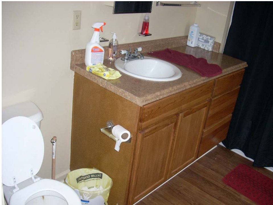
View of Bath – One-Bedroom Unit
