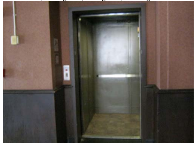
Main elevator (one of two)
