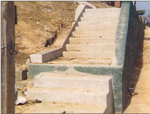
Figure 17: Photograph of concrete steps installed by MHA in March 1970 at Building 73 to combat erosion and facilitate pedestrian movement through the site. Courtesy of the Macon Housing Authority Archives.
