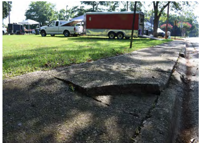
Picture 10: Cracked sidewalk in Forsyth
