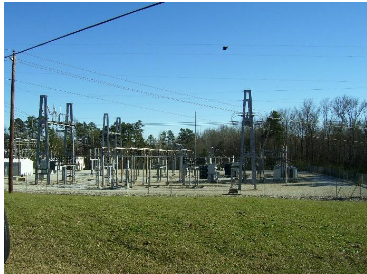
Electric Utility Substation
