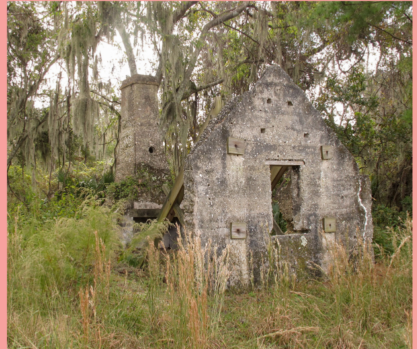
Remnants of tabby Chocolate Plantation labor site slave dwelling, Sapelo Island, McIntosh County. Ethos Preservation .
