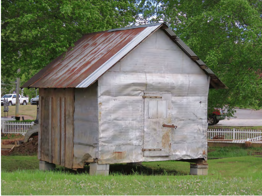
Photo 51 - View Looking South to Old Jail, Resource No. 63 (Relocated From Resource No. 49)
