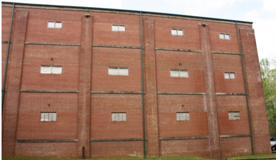
Figure 13: Photographer facing south, Photograph of Tallapoosa Cotton Mill 1948 Addition. Tallapoosa, Haralson County, Georgia, Photograph in possession of author, taken April 12, 2011. The windows in the addition have been bricked in.
