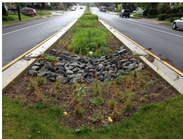
A bioswale like the photograph above is more than just a landscaped ditch. The swale should incorporate soil with a good percolation rate as well as native plants to remove pollutants.
