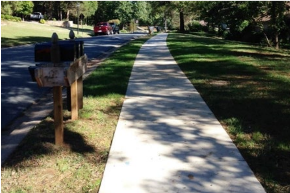
Sidewalks provide connection within a community, opportunities to exercise, and opportunities to socialize creating a more cohesive community network.
