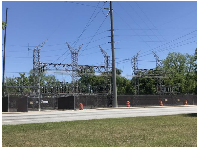
Transformer south of the Subject site
