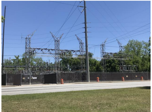
Transformer south of the Subject site
