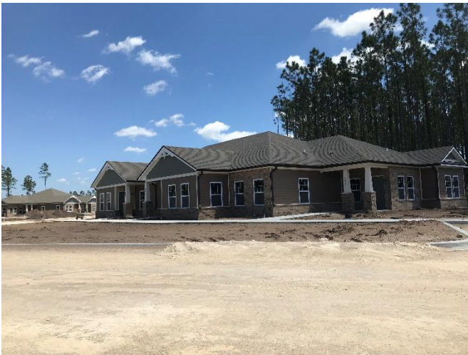
The Village at Winding Road II - Under construction east of the Subject site
