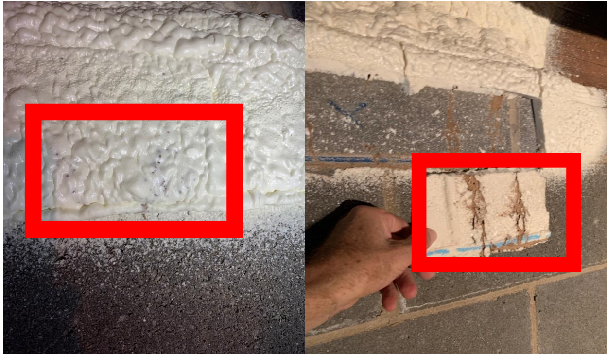
Picture 4. Images of the area in the SPF at Location 5 that provided visible evidence of termite activity on surface of SPF... left (outlined by the red box) and that same area exposed during foam removal.
