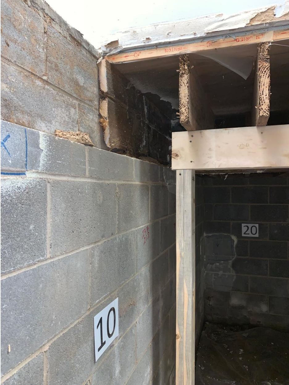
Photograph 2. Pictures of the floor joists between Locations 10 & 15 exposed during renovations conducted 6 September 2019. Pictures of each joist are arranged, left-to-right, by proximity to the joist header (on the left in this image) along the south wall of the crawlspace.
