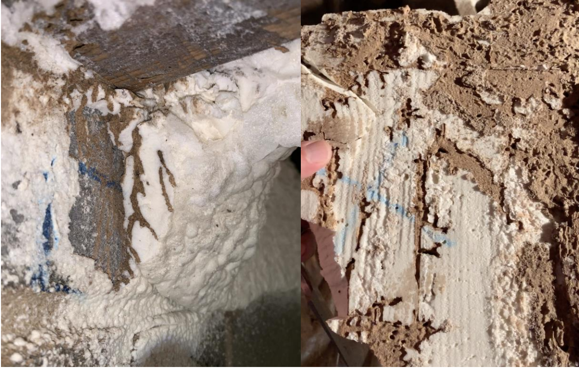
Photograph 3. Images of termite activity in the SPF observed during the August inspection from the joists and joist header by Location 5.
